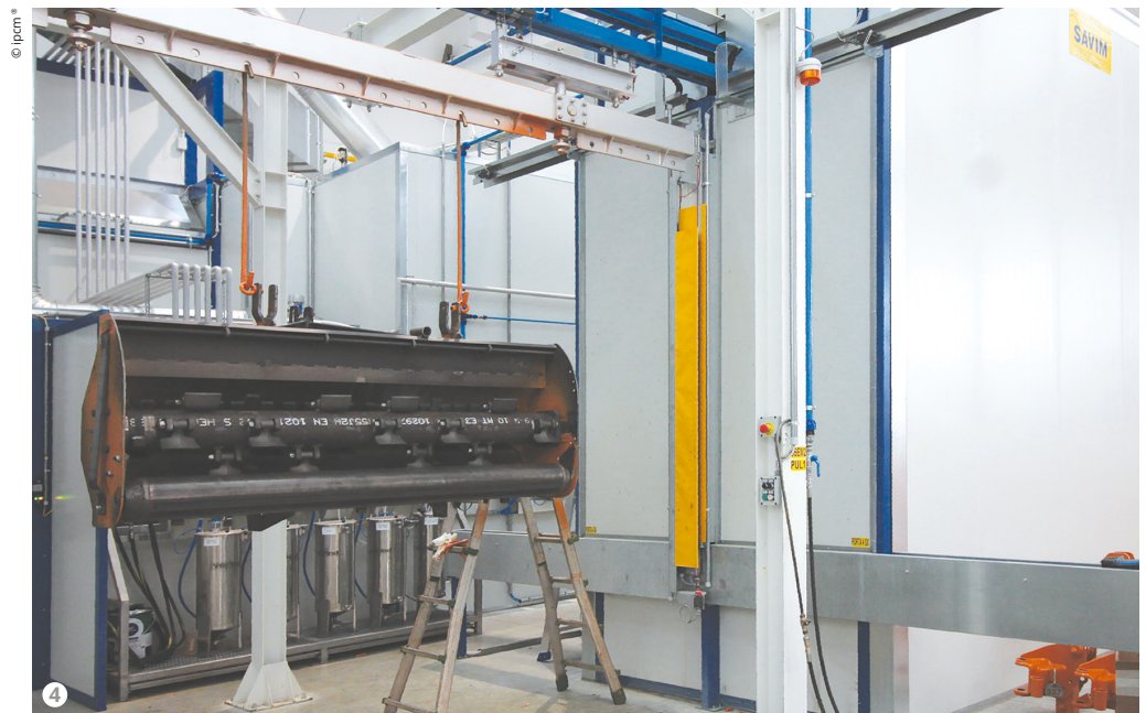
Figure 4: A component at the entrance of the pre-treatment booth.
