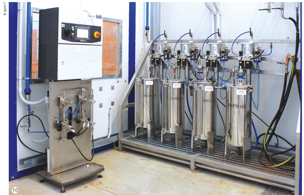
Figure 10: The coating management unit for manual station with Dürer pump.
