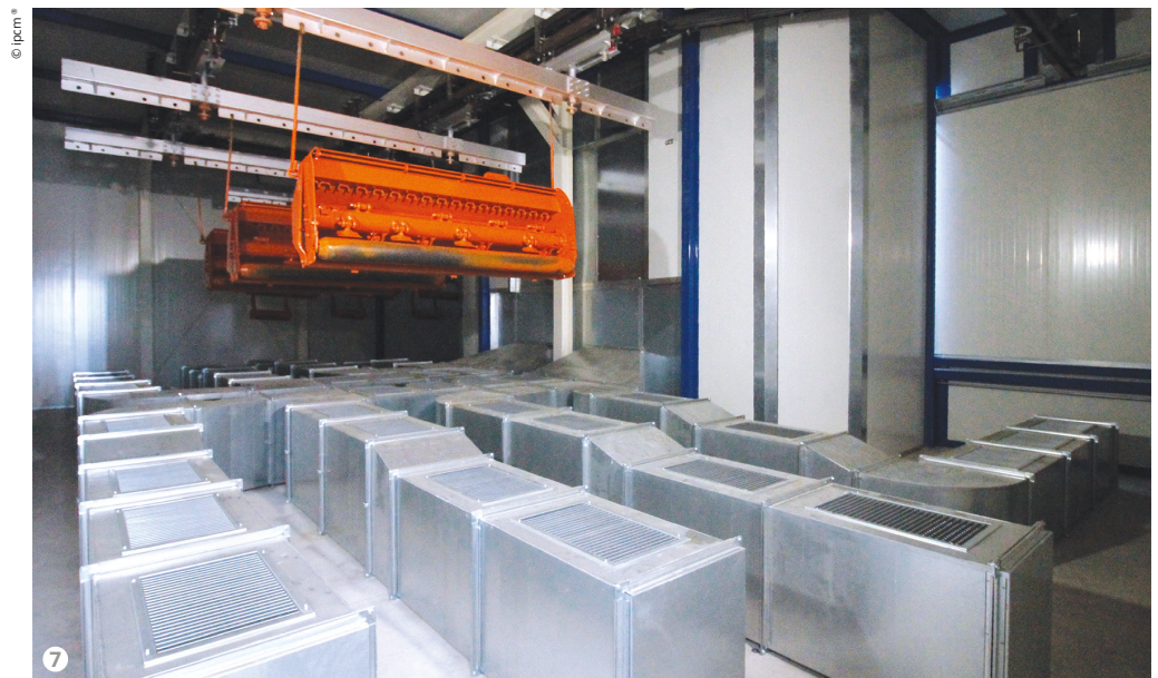
Figure 7: The curing stage in the direct fired furnace.
