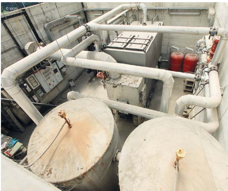
The biomass power plant.
