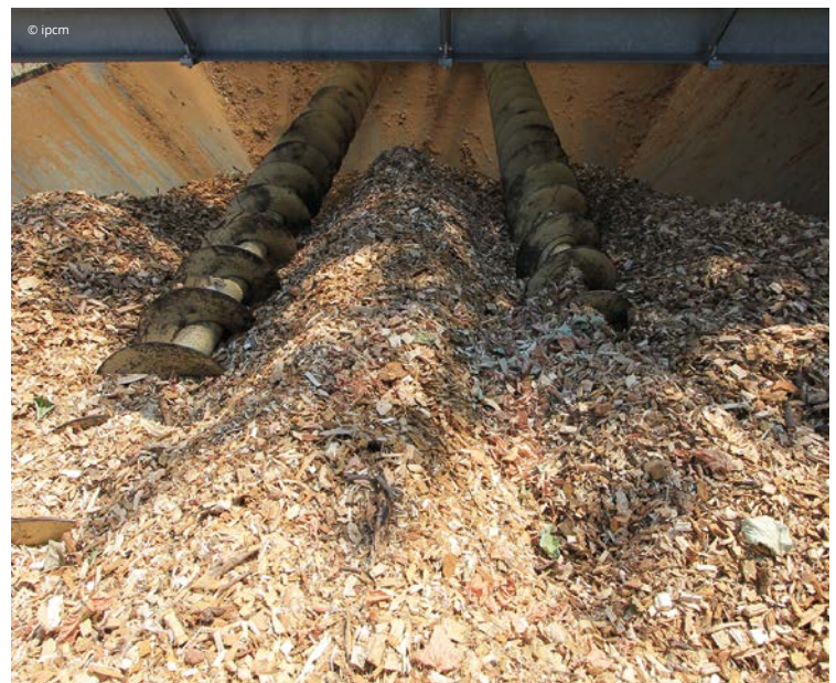
Wood chips are the Frandent plant’s heat source.
