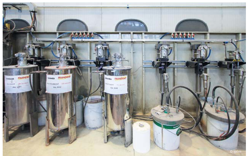
From top to bottom: The 4-stage pre-treatment tunnel, primed components, and the paint management unit.
