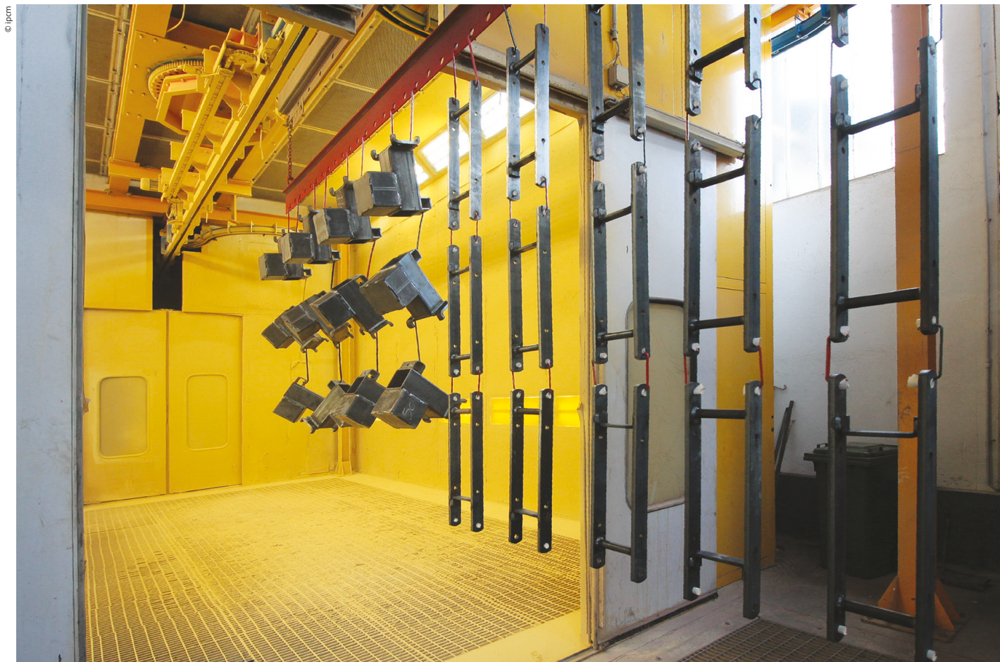
Figure 5: Workpieces exiting the coating booth, ready to be transferred to the polymerisation oven.
