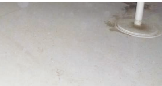
Dura-Plate UHS 600–750 microns DFT after nearly nine years of crude/water immersion
