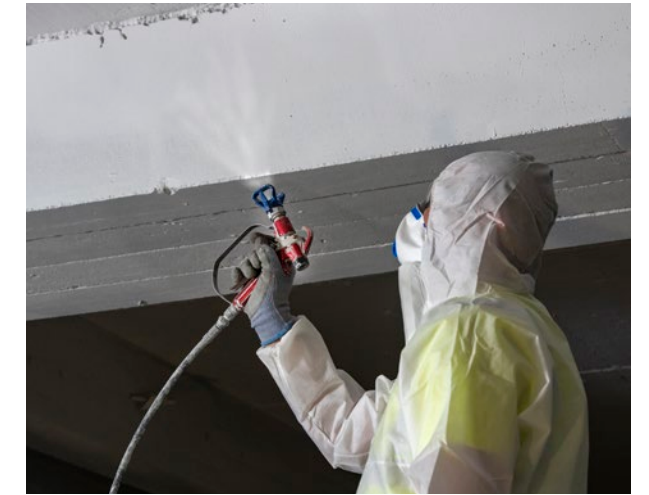
It was applied directly to the concrete ceiling using an airless spray application method.
