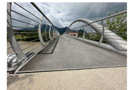
The RHD surface of the heated pedestrian and cycle bridge in Marquartstein is completely intact even after a service life of 12 years.
