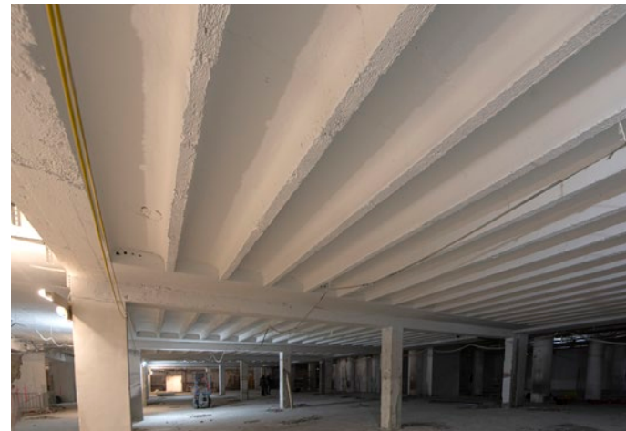
FIRETEX Concrete WB was used on an area of approx. 6,500 m 2 of Terminal 2 at Vienna airport.
