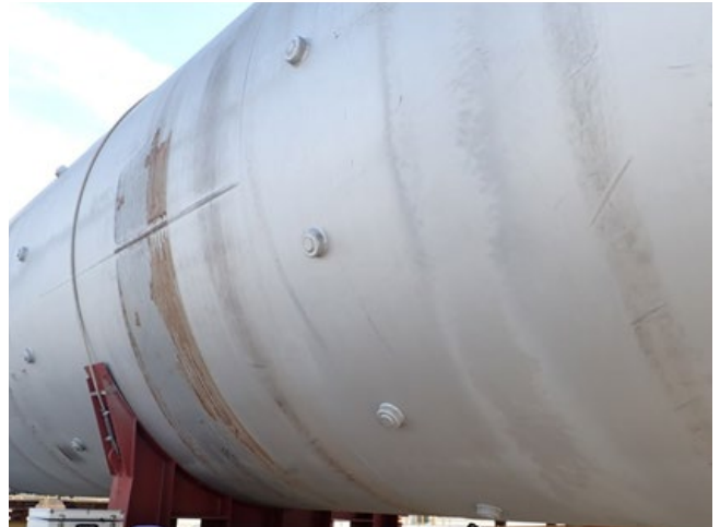
Mechanical damage typical IMM/IC Coatings
