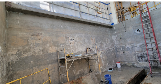
Figure 3. Crews used vertical mortars and cementitious materials to repair damaged areas and restore the original substrate profile.
