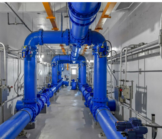
Figure 8. The rehab also included upgrades to the pipe gallery, where crews used high-pressure washing and electric bristle blasters to remove corrosion while protecting sensitive equipment.
