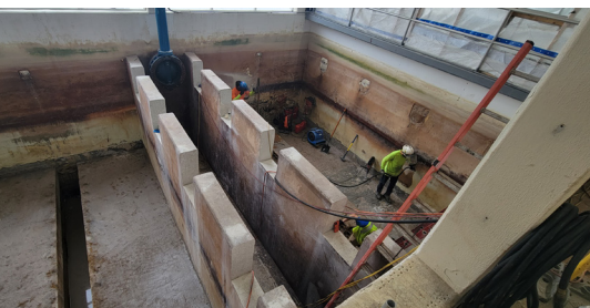
Figure 5. Applicators hand-applied Dura-Plate® 2300 at an average thickness of 3/16 inch, forming a durable base for the new coatings.
