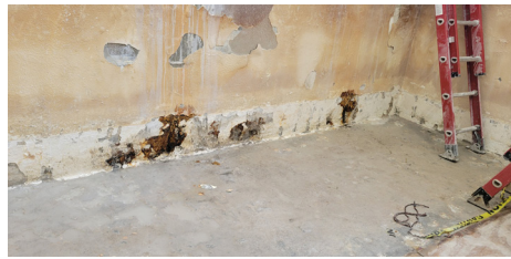
Figure 4. In newer basins with thinner coatings, surface grinding and rapid-cure mortars addressed high areas, exposed rebar and deeper damage.
