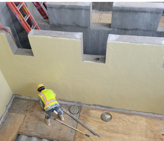
Figure 6. Final coatings included multiple layers of Macropoxy® 5500 for durability, with Pro Industrial™ epoxy applied on moisture-prone surfaces for breathable, uniform protection.
