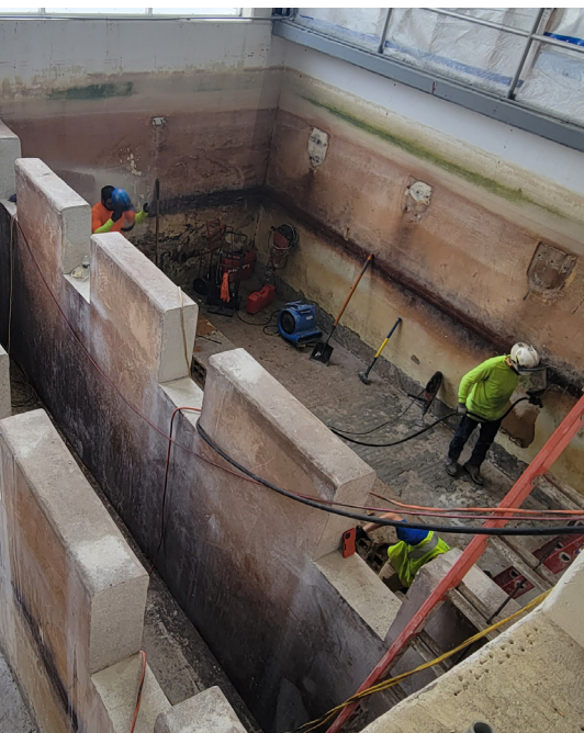
Figure 2. Crews stripped coatings to bare concrete using saw-cutting, chipping and blasting, followed by pressure washing to prepare the basins for resurfacing.
