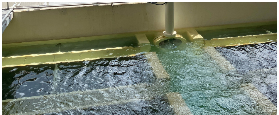
Figure 7. Each basin took about three weeks to return to service, including surface prep, equipment installation, filtration media setup and thorough holiday testing for coating flaws.
