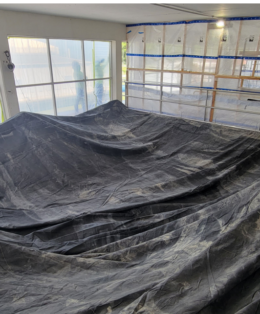
Figure 9. Custom containment structures were built around each basin to prevent contamination, with daily inspections for compliance.
