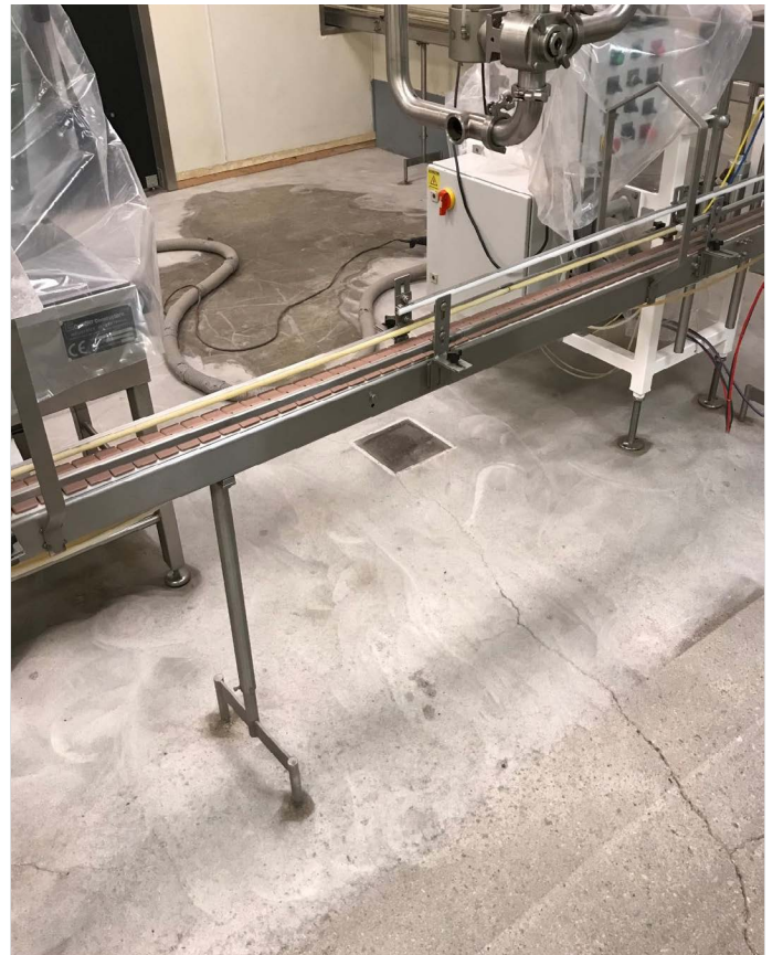
Concrete cracks may occur anywhere throughout food and beverage facilities and should be addressed using the proper repair techniques depending on the type of crack that exists.
