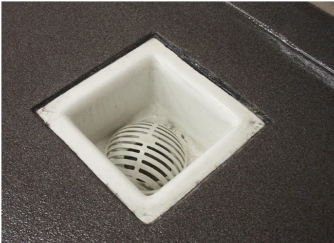
Figure 3. Infrastructure details such as drainage design and coating integrity around drains are commonly identified during a site evaluation. Addressing these items proactively helps facilities stay ahead of regulatory and environmental health and safety requirements.
