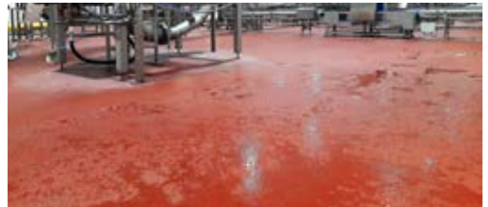
Figure 3. Wet processing areas require flooring systems that are highly resistant to constant moisture exposure and aggressive cleaning protocols. Such systems often feature textured finishes to enhance slip resistance and reduce the risk of slips and falls.
