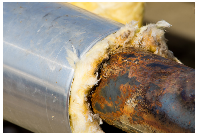
Figure 2. Eating away at steel substrates, CUI may eventually weaken the metal and cause dangerous leaks or explosions to occur.
