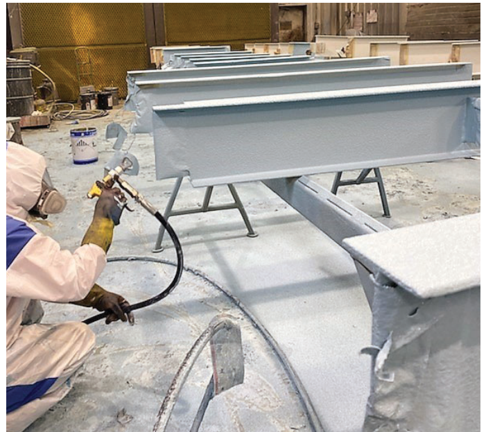
Figure 2. Applying IFRMs at ground level in a shop enables safer and more accurate fireproofing applications, while also minimizing on-site coatings activities so applicators can minimize disruptions to other trades working at the jobsite.
