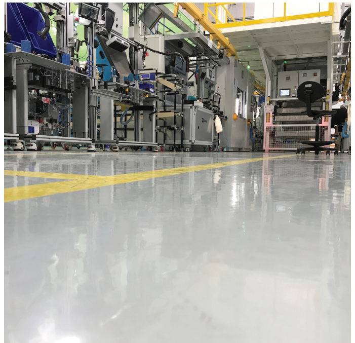
Figure 3. Poured-in-place high-performance resinous flooring creates a smooth, seamless surface that doesn't shed particulates, making it ideal for meeting the clean room-level requirements of data centers.
