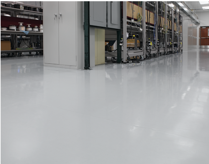
Figure 4. Data center areas housing sensitive microelectronics require ESD flooring to prevent even tiny static shocks from harming equipment.
