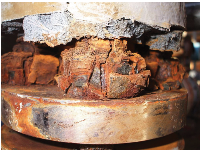
Figure 1. Corrosion under insulation (CUI) is a bane of many energy-related applications that can be mitigated or eliminated by optimizing coating selections at the outset of a project.
