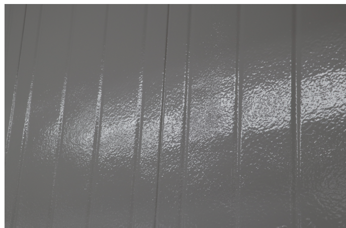
Figure 1. Close-up of an IMP wall surface after resinous coating application. The system bridges panel seams and creates a continuous, cleanable finish that reduces areas where moisture can collect.
