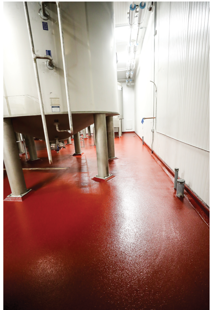
Figure 4. A food and beverage processing area showing a resinous floor system with a cove base transition to IMP walls. This type of interface would be assessed for cleaning access and moisture risk during a site evaluation.
