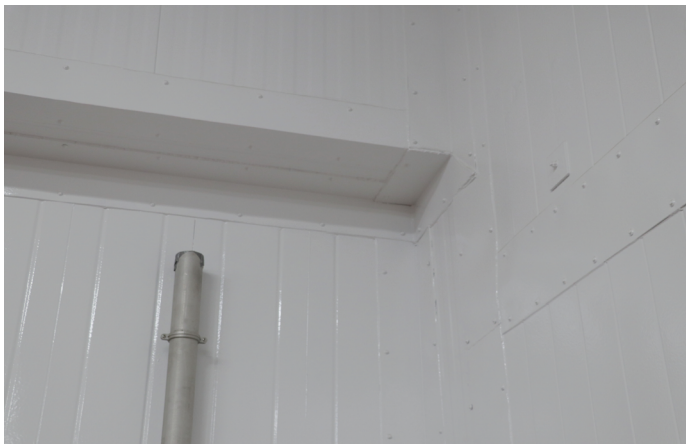
Figure 2. Detail view of a coated IMP wall showing how resinous systems can cover seams, corners and transitions with a more continuous finish. These areas are often the first places where conventional sealants and patch repairs begin to fail.
