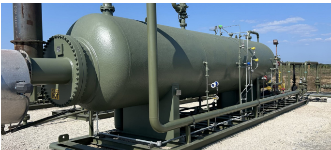
Figure 4. While not part of pipeline infrastructure, this heater treater is a representative example of how TICs can replace traditional insulation systems. The unit was first primed with Heat-Flex® ACE for corrosion protection (top) and then covered with the TIC Heat-Flex® Advanced Energy Barrier (middle) to lock in process heat with no physical insulation system needed. Finally, applicators topcoated the unit (bottom) for aesthetic and durability purposes.
