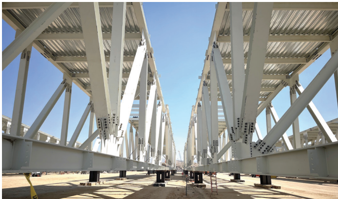
Figure 2. Structural steel used in semiconductor fab operations should be coated with CRCs that have been qualified, tested and approved for use in clean zones.
