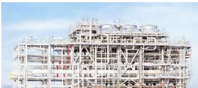
Figure 1. A variety of stainless steel assets exposed to cryogenic service and highly corrosive environments in LNG operations are often insulated, elevating the risks for corrosion under insulation (CUI) to develop and proliferate.
