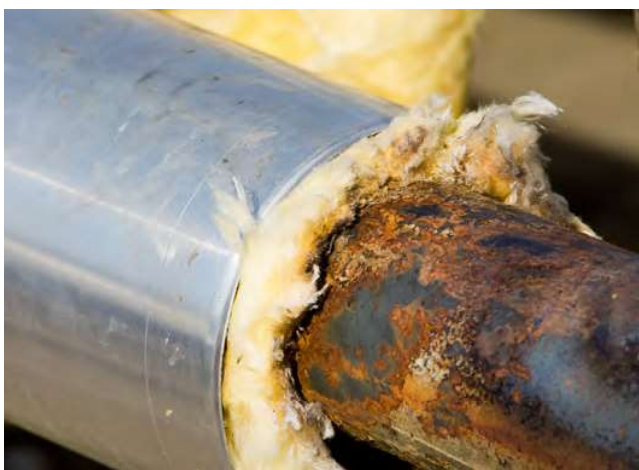
Figure 2. CUI can eat away at steel substrates, leading to weakening of the metal to the point that dangerous leaks or explosions may occur.
