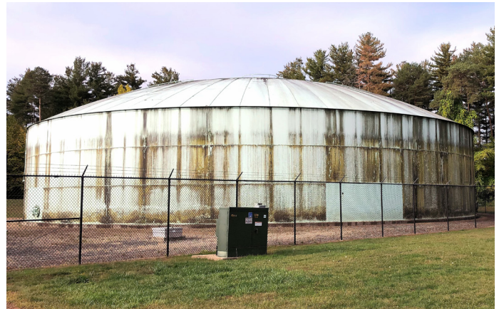
Figure 5. This water storage tank exterior showed widespread surface contamination and mildew buildup prior to maintenance. Image courtesy of Sherwin-Williams Protective & Marine.
