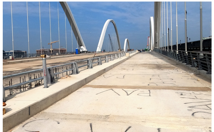
Figure 4. In-service bridge conditions can combine deicing salts with traffic-related deposits and moisture cycling — a mix that can drive cleaning demands and influence long-term coating performance. Image courtesy of Sherwin-Williams Protective & Marine.
