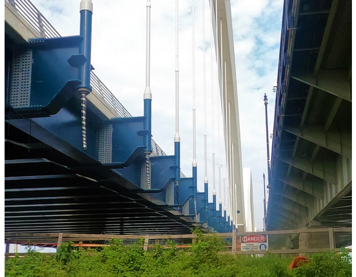
Figure 3. On the Frederick Douglass Memorial Bridge steel, the organic zinc primer's shorter recoat window supported quicker topcoating and fewer hold points in the two-coat workflow. Image courtesy of Sherwin-Williams Protective & Marine.
