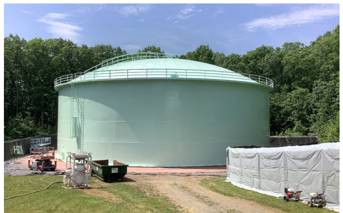
Figure 6. After recoating the tank with a Sher-Loxane® 800 finish, it features a restored appearance that will support long-term cleanliness. Image courtesy of Champion Painting.
