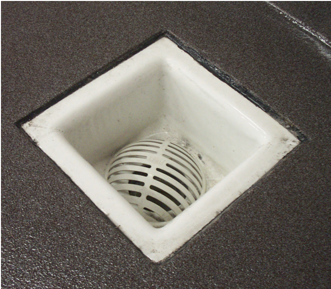
Figure 3. A coatings professional may recommend that a facility convert longer trench drains into box drains (shown) to reduce the amount of surface area where microbes can become trapped and promote bacteria growth.
