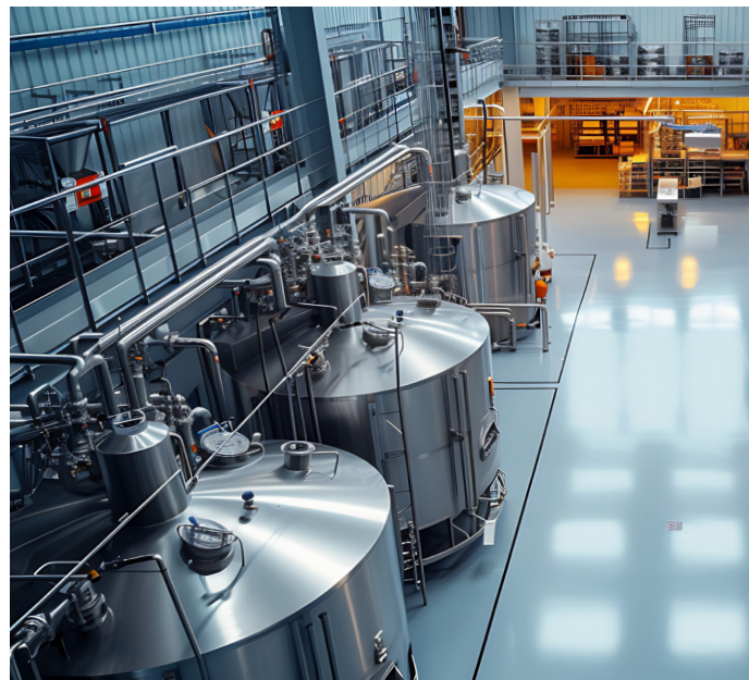
Figure 1. During a facility evaluation, a coatings professional will cover the entire site looking for any potential deficiencies such as corrosion, peeling paint, cracked flooring, and porous surfaces that can harbor bacteria.
