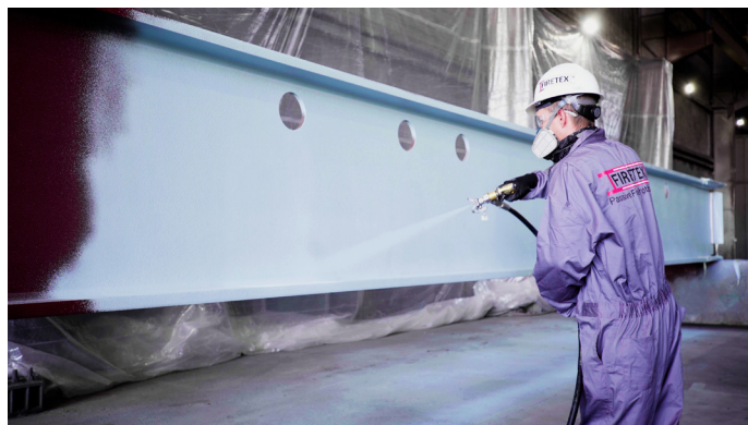
Figure 6. Applying epoxy intumescent fireproofing off-site before constructing a cleanroom environment removes a host of on-site challenges.
