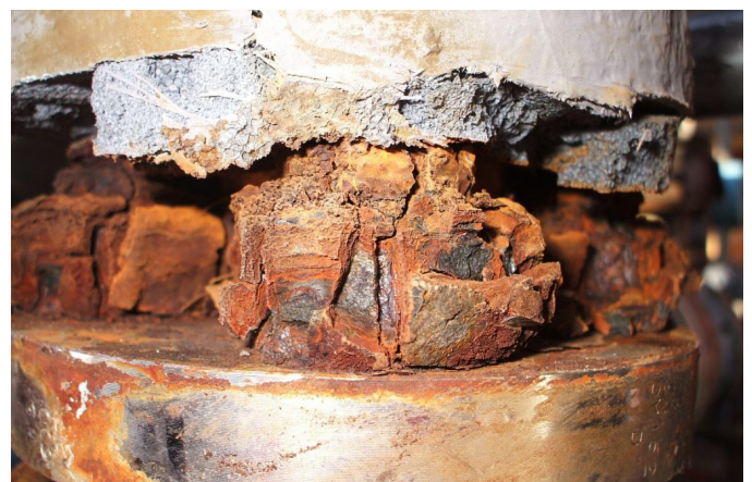
Figure 1. Although pipes and other assets are coated prior to being covered with insulation, CUI is inevitable over time. Choosing an optimal coating system that mitigates CUI will slow down that process, providing longer service lives and reduced ownership costs.
