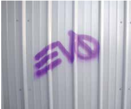
BEFORE: Spray paint graffiti markings on surface coated with Sherwin-Williams Coil Coatings’ ASTM-compliant coating.
