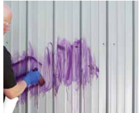
AFTER: Cleaning with GRS non-toxic solution, the surface will look new with no coating damage within a few minutes.
